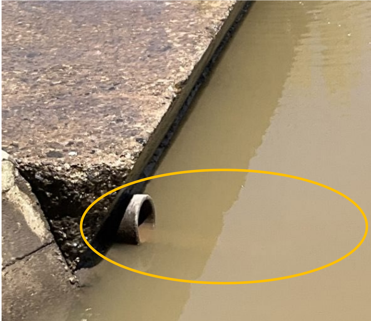
Soil coming out of a drain under the service spillway.
