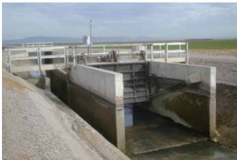
Radial Gate Structure 3 on main canal
