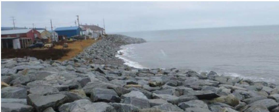
Coastline eroding along Native Alaskan village
