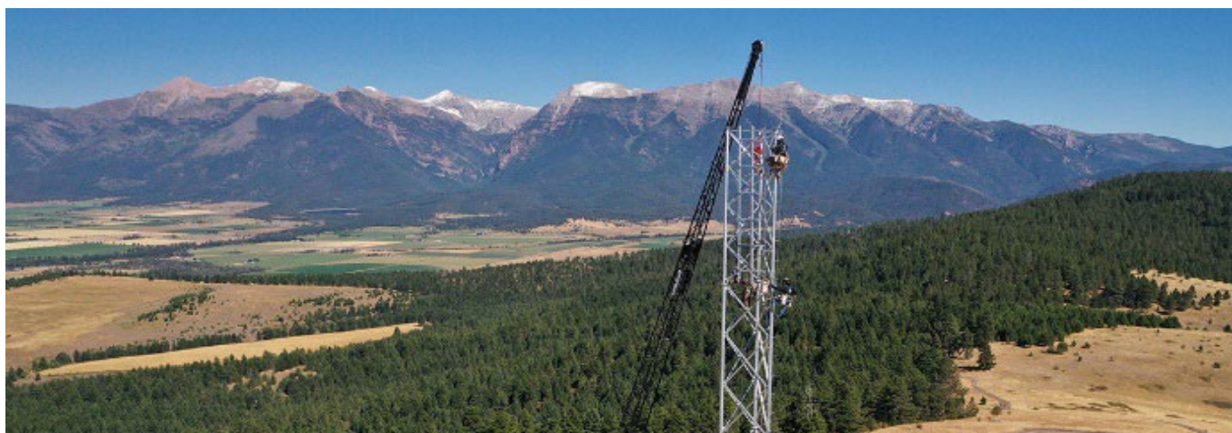
Salish Kootenai Tribe (SKT) Broadband Tower Project on the Flathead Reservation
