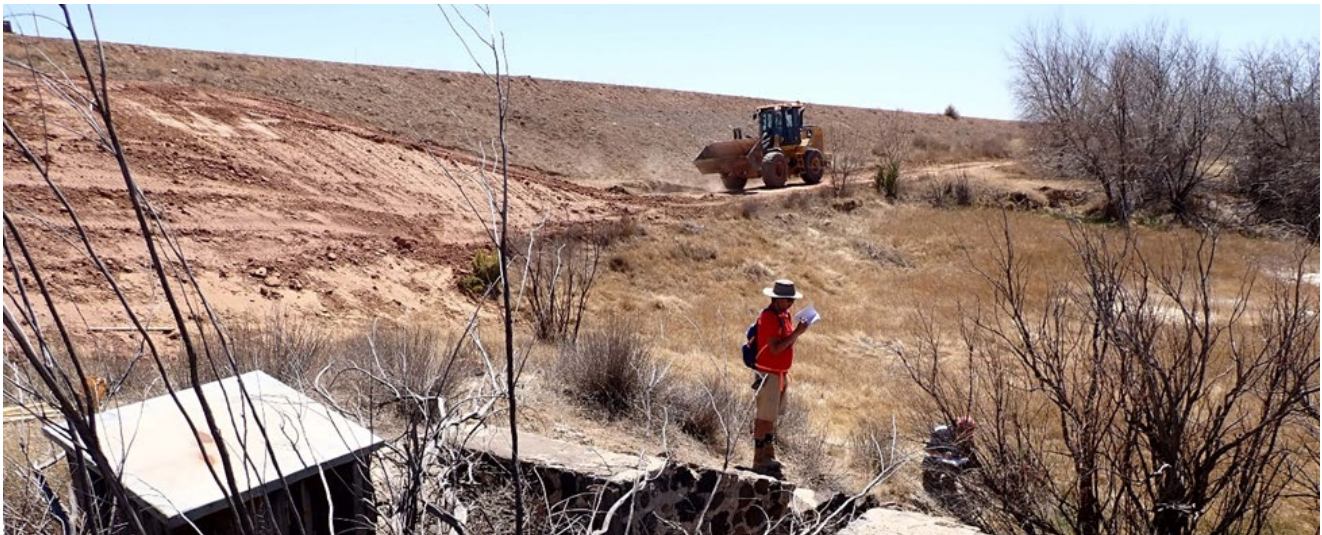
Laguna Tribal Historic Preservation Office (THPO) staff and the SW Regional Archaeologist record an abandoned operational feature of the Mesita Dam. The buttressing dirt beam is on the upper left with heavy equipment stabilizing the dam in the background.
