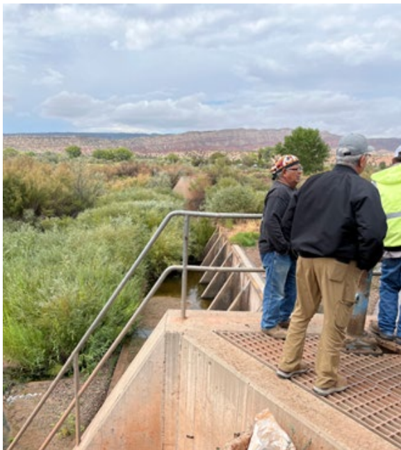
Lt. Governor Benjamin R. Salas of Zia and Tribal Council member surveying damage to irrigation dam after the flood
