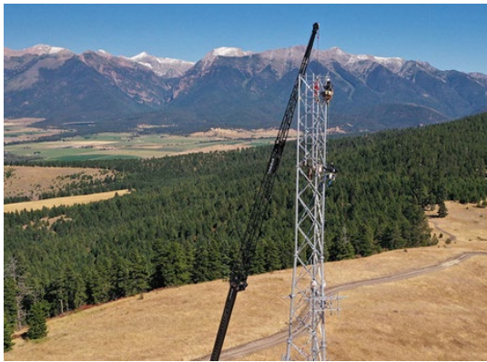
Installation of 2.5 GHz radio frequency band tower to provide broadband services on the Flathead Reservation
