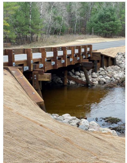
Broomhead Road timber bridge crossing of the Ottaway (Boardman) River installed in 2022.
