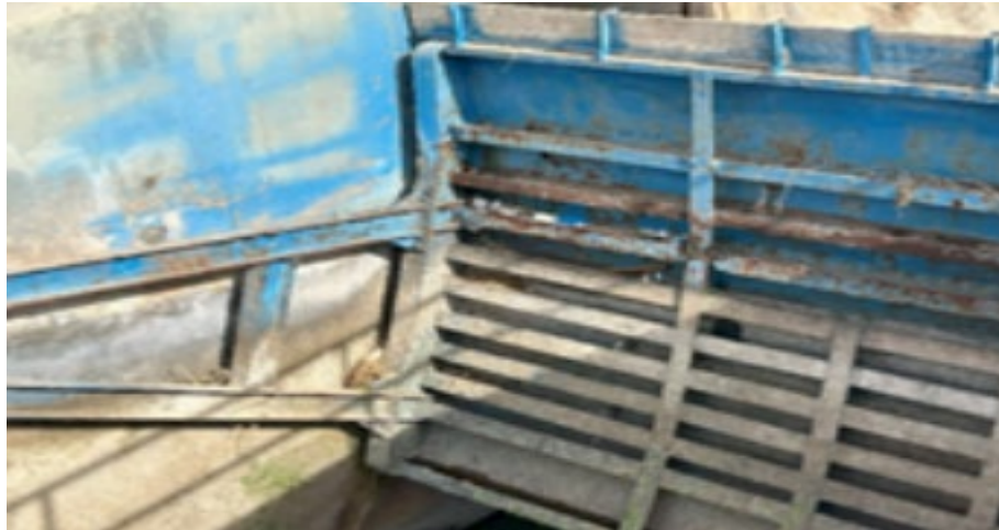
CRIP Headworks Radial Gate
