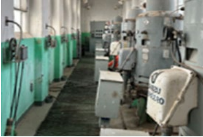
Fort Hall Pumping Plant Interior of Bannock Pumping Plant
