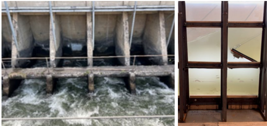
Photo 1: Damaged Concrete at Wapato Headgates; Photo 2: Wapato Diversion Dam Sectional Headgate Model with Juvenile Salmon
