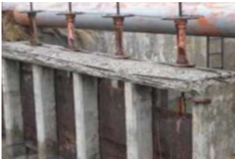
Fort Hall Deteriorating Concrete at the Reservation Main Headgate
