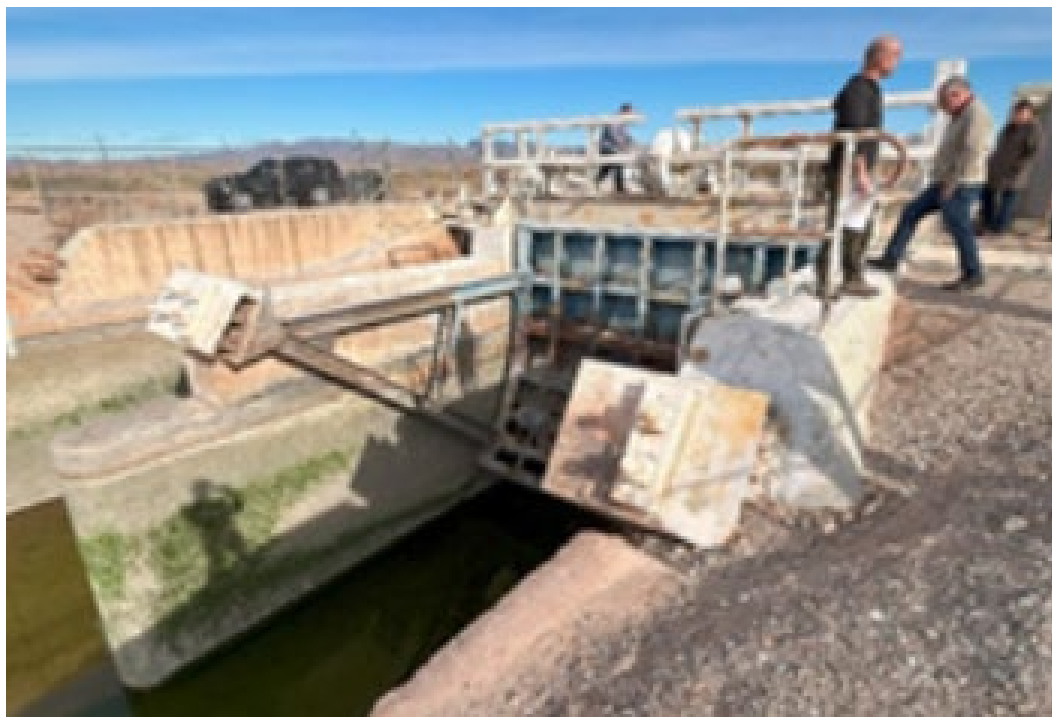
CRIIP Radial gate at Main Canal Check 420
