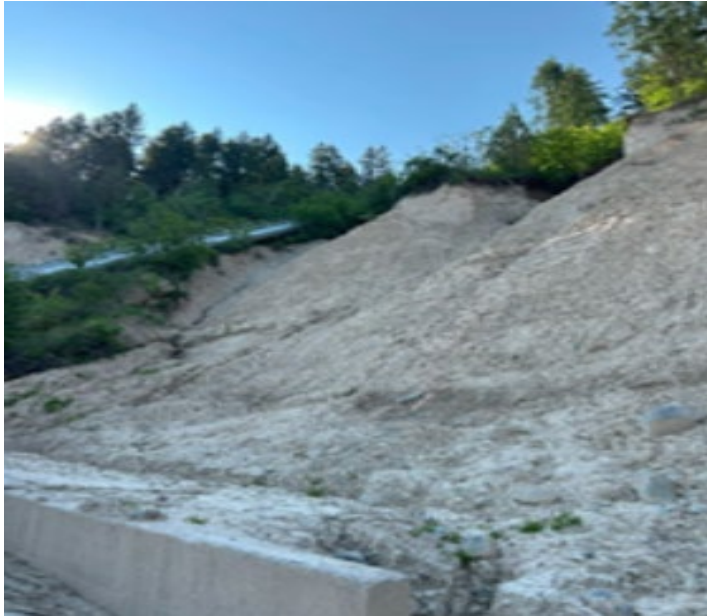
Flathead Pumping Plant Erosion Adjacent to and Beneath Penstocks
