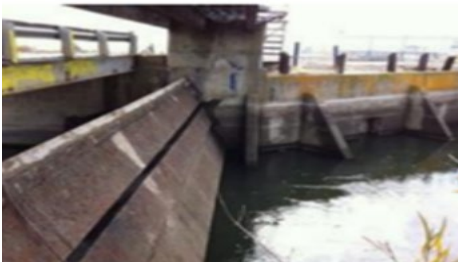
Satus Main Headgate Prior to Failure
