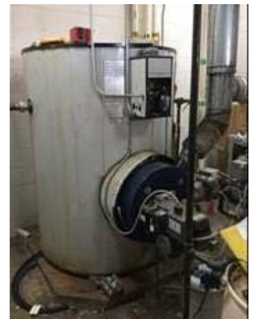
Boiler at Blackfeet Dormitory in Montana
