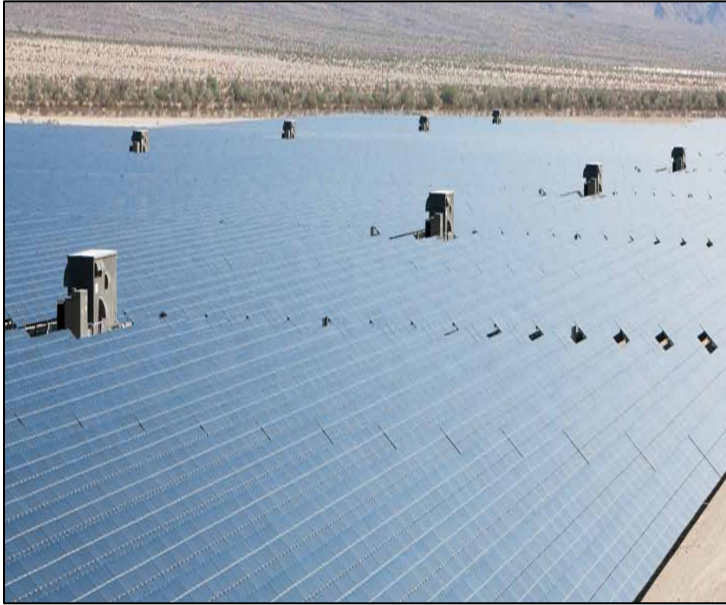
Figure 11. Moapa Band of Paiute Indians utility scale solar project.
