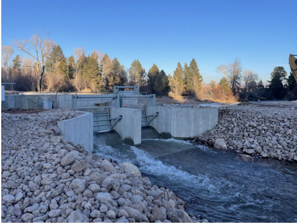
Uintah River bifurcation replacement, Uintah Indian Irrigation Project, Utah – construction complete – radial gates shown are about 4 feet tall.
