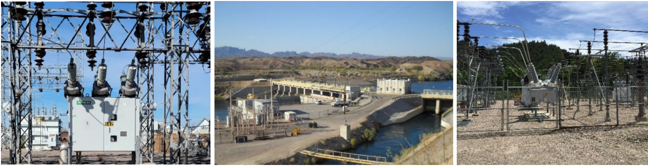
Transmission breaker at Coolidge Substation, AZ; Powe Generation Facility at Headgate Rock Dam, AZ/CA border; Kerr Substation, MT
