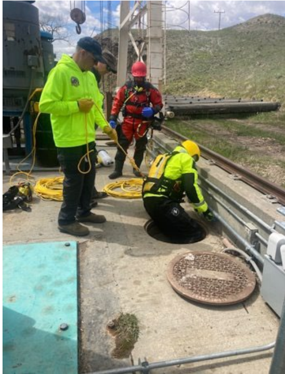
Wiota Pumping Plant at Fort Peck Indian Project, Montana – divers implementing pumps and impellers.
