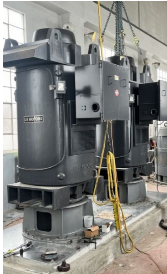
Portneuf Pumping Plant at Fort Hall Indian Irrigation Project, Idaho – new pumps installed.
