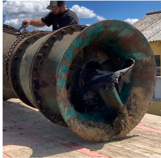
Wiota Pumping Plant at Fort Peck Indian Project, Montana – belt wrapped around impellar.
