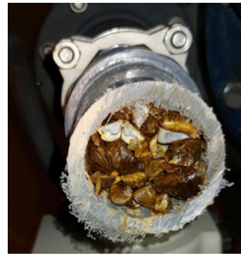
Damages water and power delivery systems (invasive mussels)
