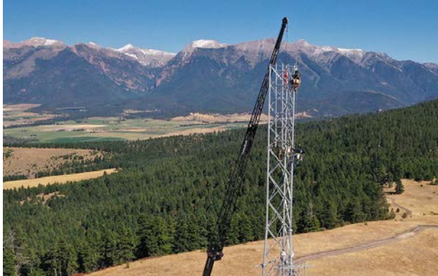
Installation of 2.5 GHz radio frequency band tower to provide broadband services on the Flathead Reservation
