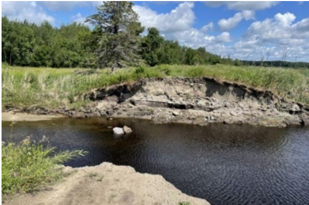
Breach of Kiwosay Dam, Red Lake Reservation, MN
