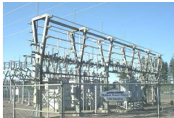
Mission Valley Power, Kerr Substation
