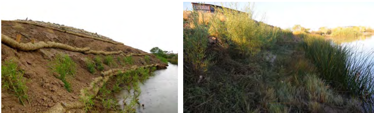
Figure 10-2. Bundles of fast growing plants planted along the bankline can help provide erosion control when steep banks cannot be re-graded. Left: grass bundles installed along a steep bank with willow bundles planted in between to stabilize and capture soils on the bankline. Right: The same bankline one year later. Photos courtesy of Fred Phillips Consulting.
