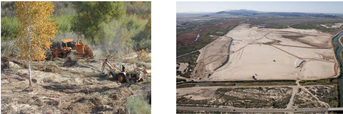
Figure 9-1. Examples of mechanical treatments. (Left) Tractors grubbing root systems for large tamarisk stands. (Right) A site cleared of invasive tamarisk using mechanical treatments. Photos courtesy of Fred Phillips Consulting, LLC.
