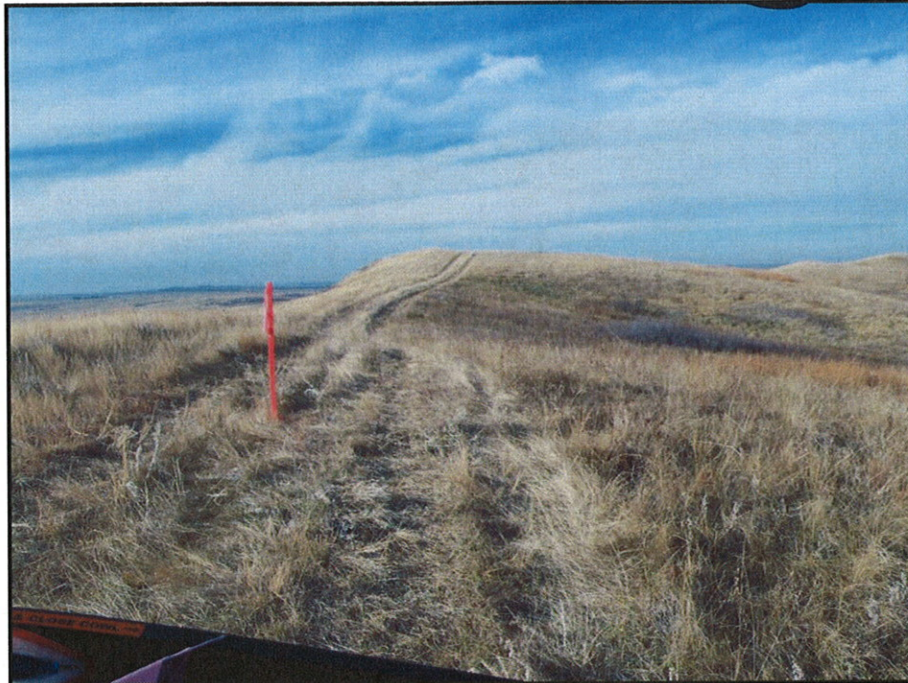
Figure 9. Construction access two-track road. Photo taken facing west, as pipeline will cross ridgeline.
