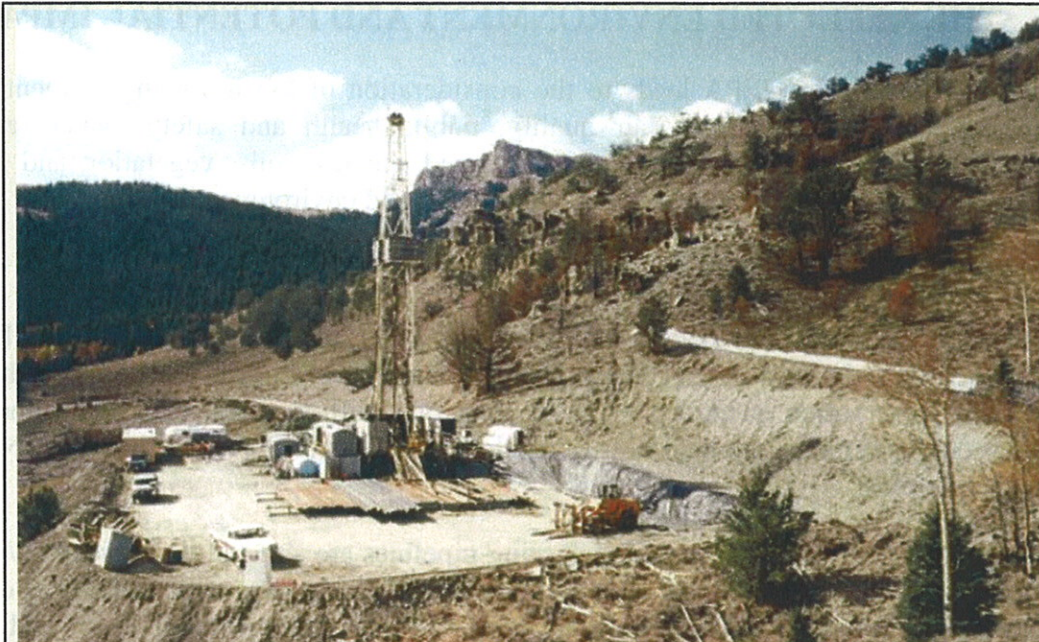
The well pad and access road are constructed to the minimum size necessary to safely conduct drilling and completion operations.
