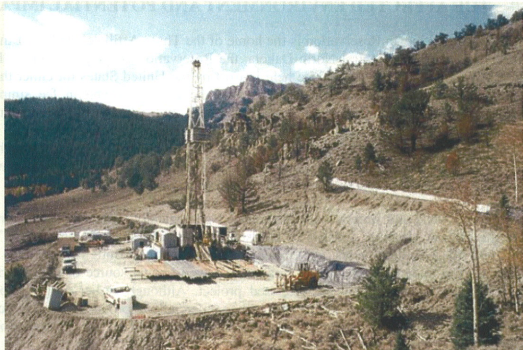
The well pad and access road are constructed to the minimum size necessary to safely conduct drilling and completion operations.
