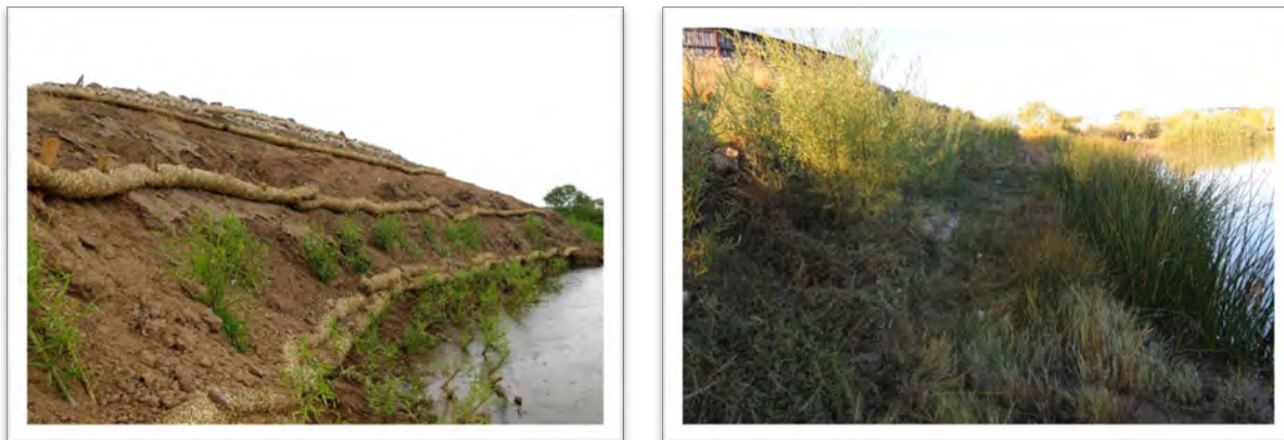
Figure 10-2. Bundles of fast-growing plants planted along the streambank can provide erosion control when steep banks cannot be re-graded. Left: grass bundles installed along a steep bank with willow bundles planted in between to stabilize and capture soils on the bankline. Right: The same bankline one year later. Photos courtesy of Fred Phillips Consulting.
