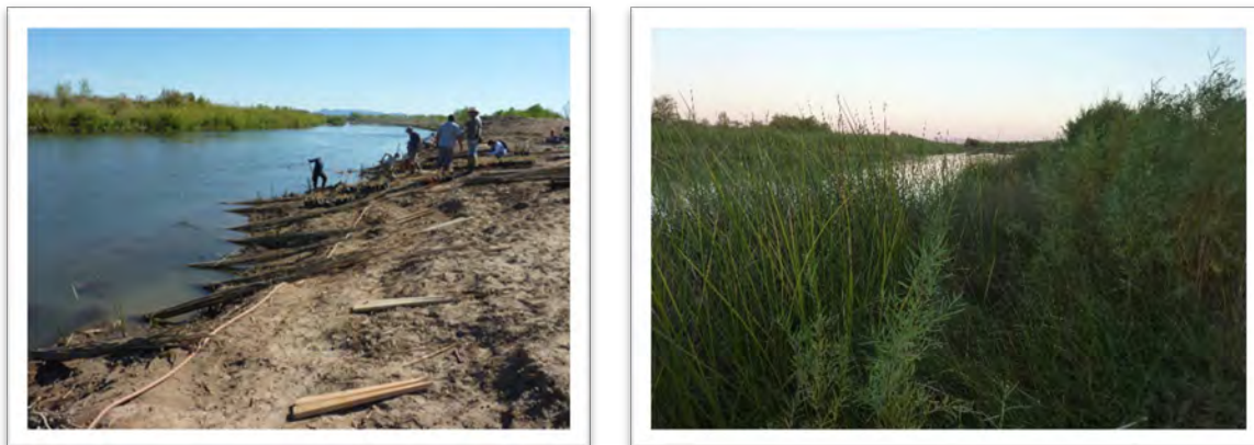
Figure 10-1. Harvested willow poles are planted along a bankline to provide additional erosion protection. Left: Work crews prep the bundles of willow poles after they have soaked in the Colorado River. Right: the same location one year after planting. Photos courtesy of Fred Phillips Consulting.
