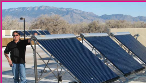
SIPI Maintenance Mechanic Bill Dyea with hot water panels.
