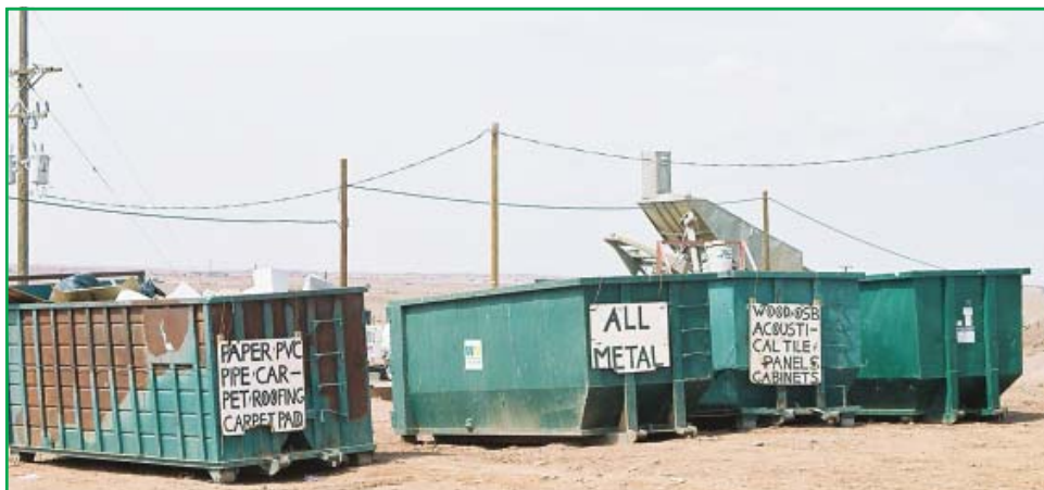
The replacement school construction site at Leupp, Ariz., featured separate bins for proper disposal of construction waste, frequently a LEED rating system point.
