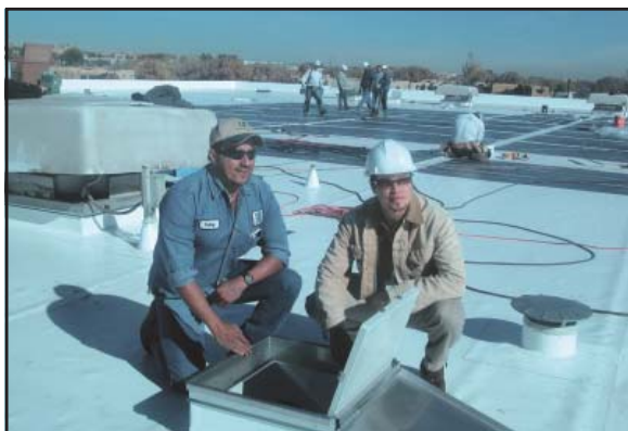
Acting SIPI Facility Manager Gary Trujillo (left), Isleta Pueblo, and OFMC Project Manager Andy Robinson, Northern Cheyenne, supervise solar collector installation.
