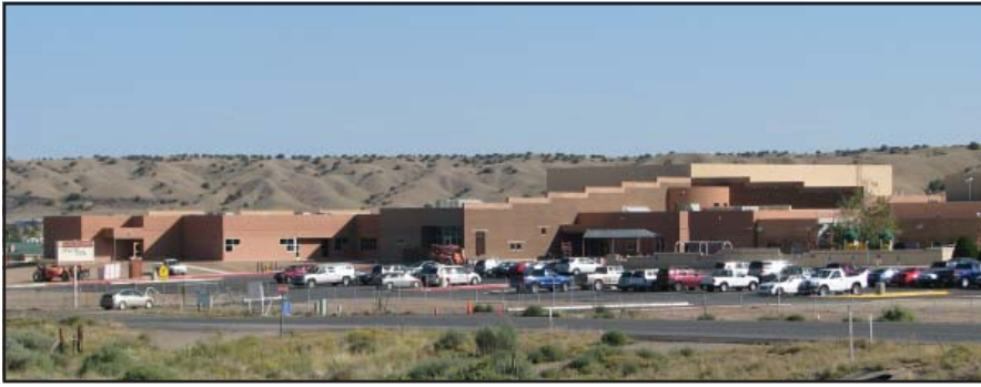
San Felipe Pueblo Elementary School gymnasium and middle school addition nears completion.
