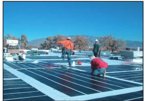
Solar collectors are installed atop the SIPI gymnasium and will also be installed atop the administration building.
