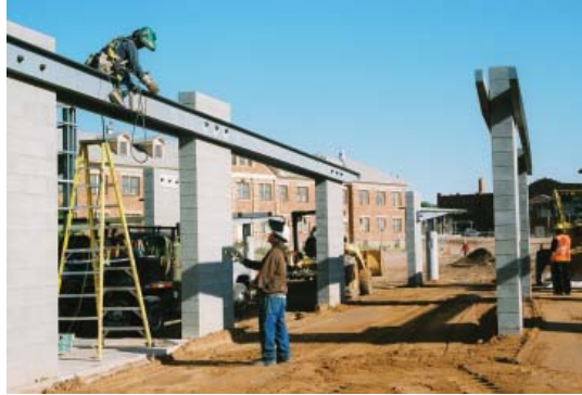
Construction workers weld girders for a new building situated near one of the five historic buildings that will remain on the campus.
