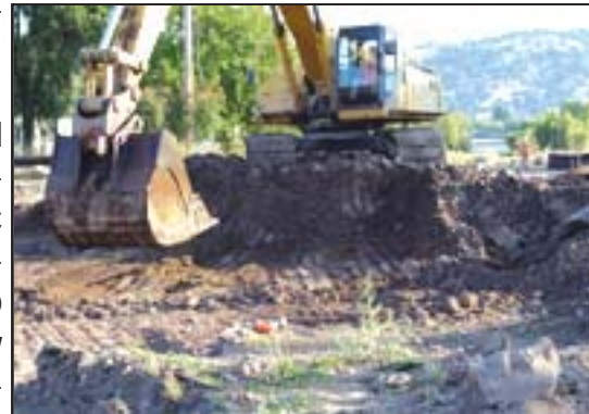
Digging several feet deep, the excavation of the subsurface of the Elem Colony's roads begins.
