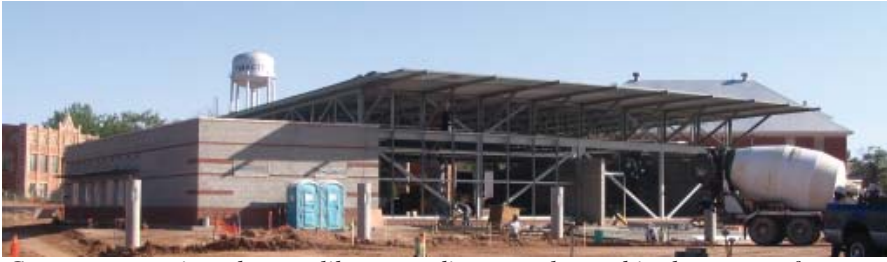
Concrete pours into the new library-media center located in the center of campus.
