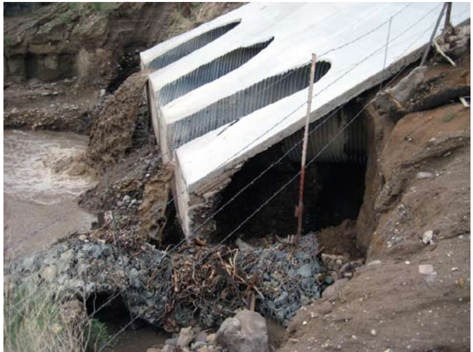
SP-90/Cochiti Hwy-Bland Canyon road crossing - downstream of culvert crossing. ~ Photo by Weiss, 2013
