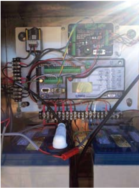
Peralta Windmill early warning system flood stage gage enclosure. ~ Photo by Weiss, 2013
