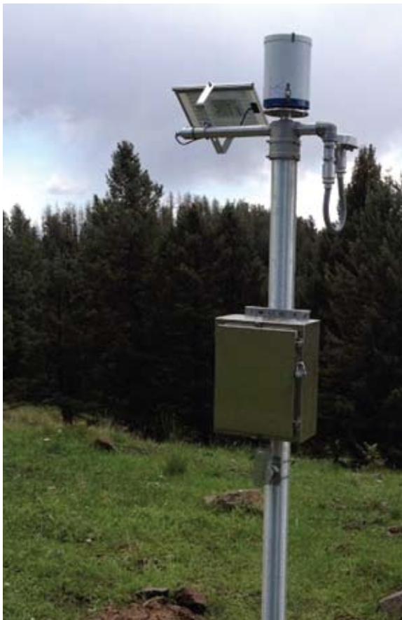
Peralta Ridge early warning system precipitation gage - completed installation ~ Photo by Weiss, 2013
