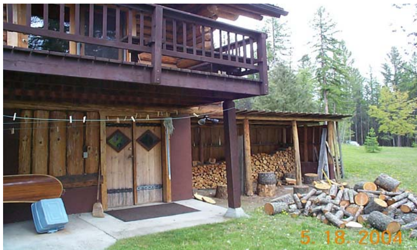
Embers can easily get underneath in this home. This house should have protection around the foundation.
