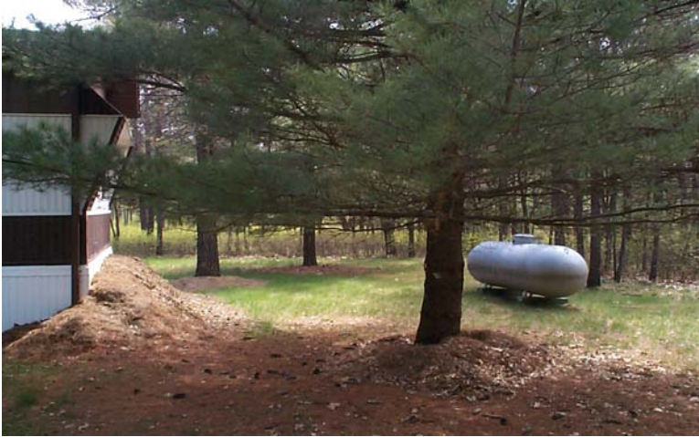
Pine needles piled against structure, tree should be limbed up.
