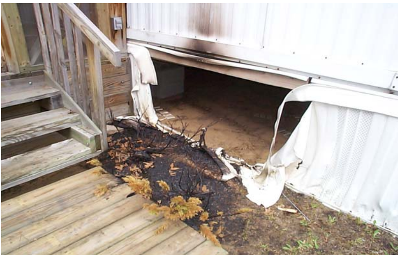
Brush against trailer skirting.
