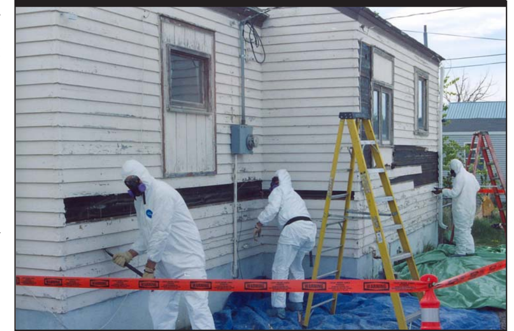
Blackfeet Tribal member John Butterfly (left) removes lead paint siding from a home in Browning Mt. Butterfly, a college student, is working on the BIA-funded project for the summer.
